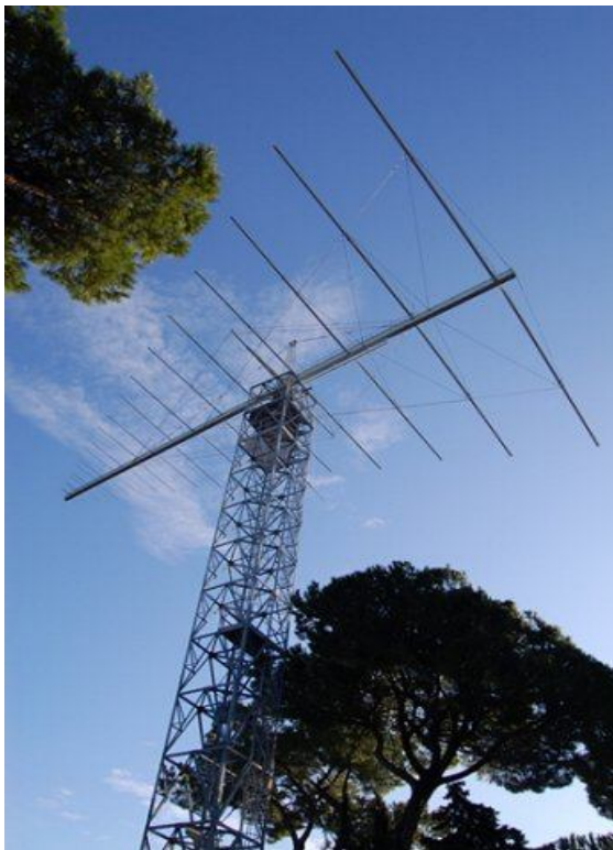
H.F. Log Periodic on Tower.
